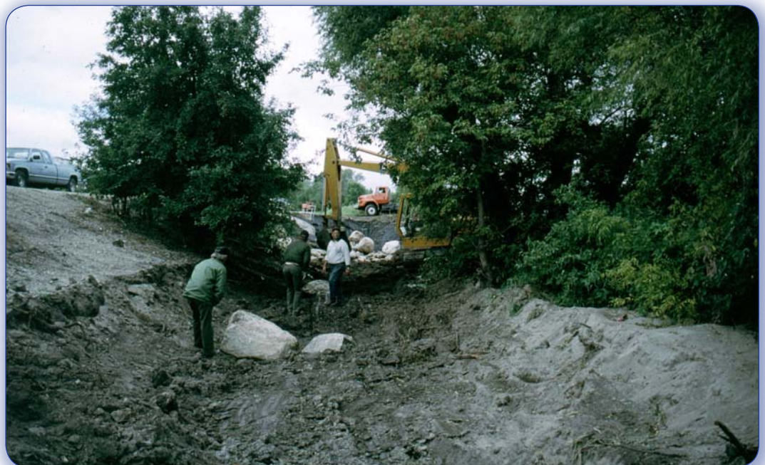
Figure 83. Construction of the Breckenridge Fishway channel showing placement of the boulder weirs.
