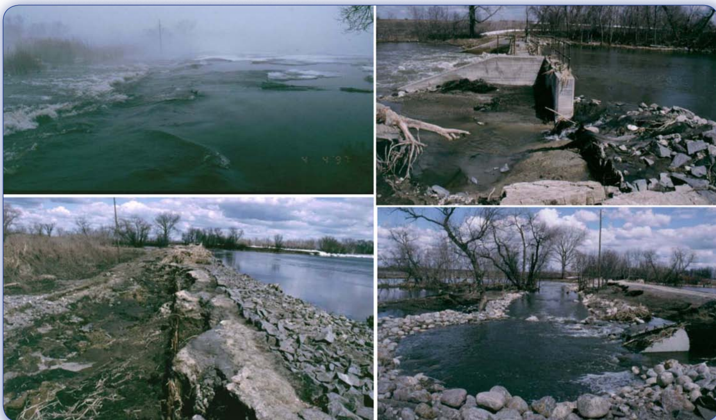
Figure 85. The 1997 flood and damage to the Breckenridge Dam.
