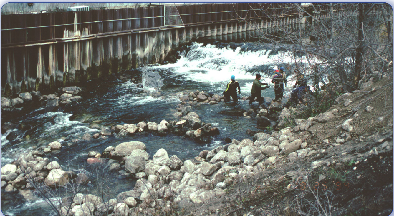
Figure 64. Hand placement of fieldstone during the initial conversion of the Steam Plant Dam to rapids, October, 1994.
