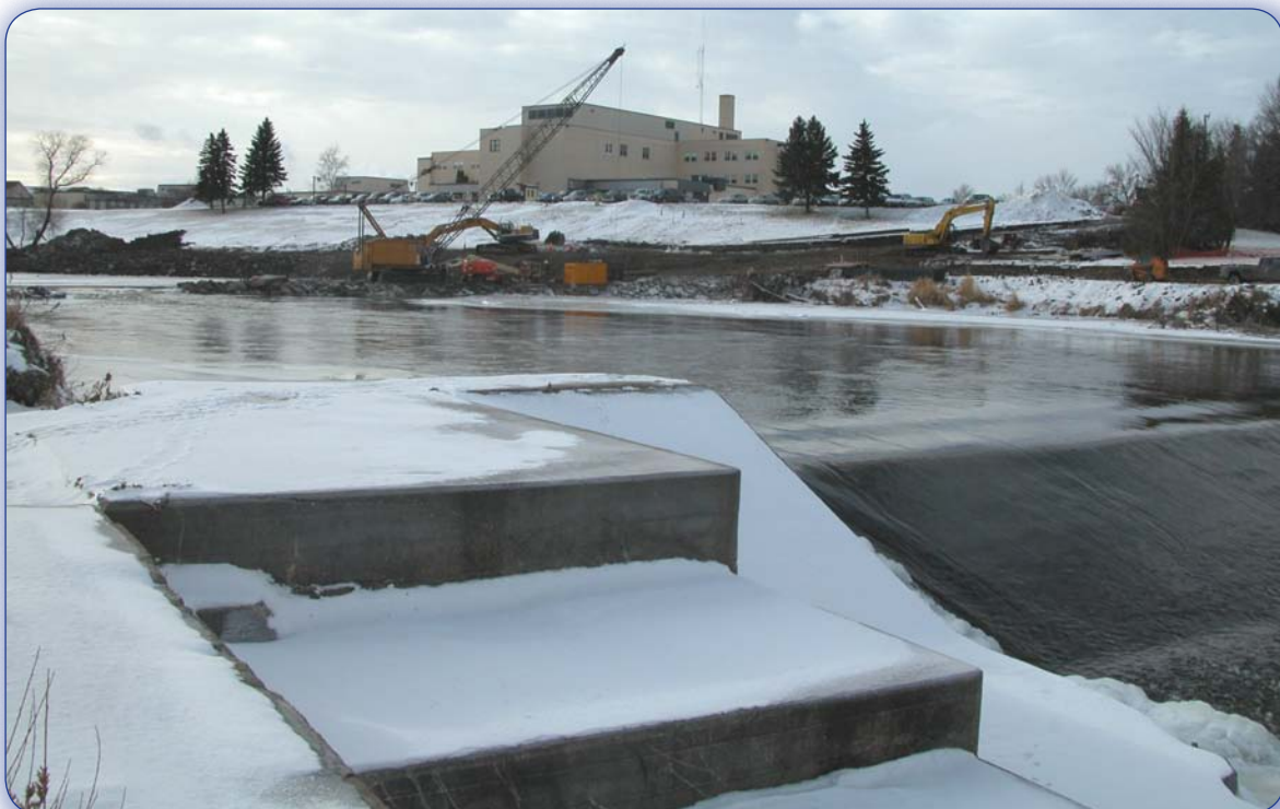
Figure 98. Construction of the rapids crest in the background and the old dam crest in the foreground.
